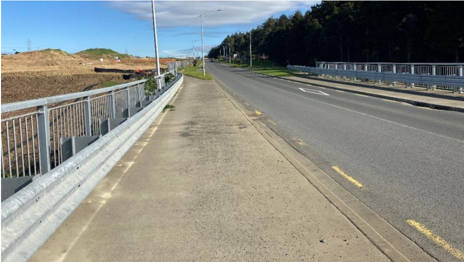
Figure 5 Murphys Park Drive (looking west from the eastern end of the bridge)
